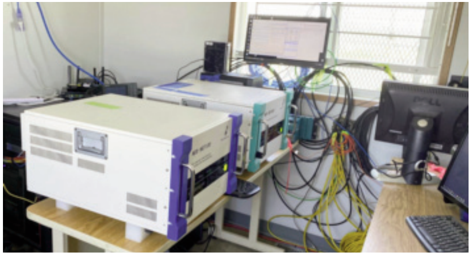
Fiber optic interrogator units that are connected to fibers that run down the wellbore for thousands of feet. Image courtesy Neubrex Ltd
