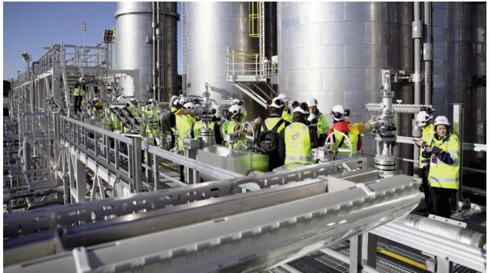
The Northern Lights Carbon Capture and Storage facilities. Photo: Torstein Lund Eik / Equinor
