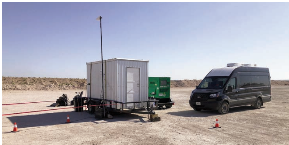
Fiber optic data acquisition units on a remote well pad location (Image courtesy Neubrex Ltd)
