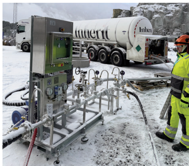
In Øygarden Inherit offloads the CO2 trucks to the tank farm from where Northern Lights transports the CO2 offshore via pipeline and will safely store it 2,600 metres below the seabed
