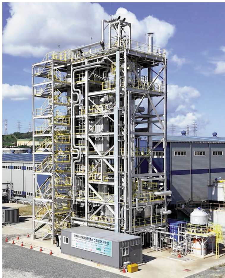
Figure 2 – 3 MW th NG-CLC steam generation plant
