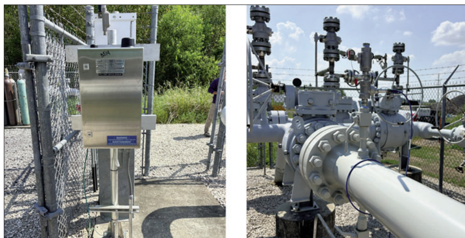
Figure 4 - PipeSense delivered a new dynamic pressure analysis-based leak detection system to a Texan sCO 2 pipeline
